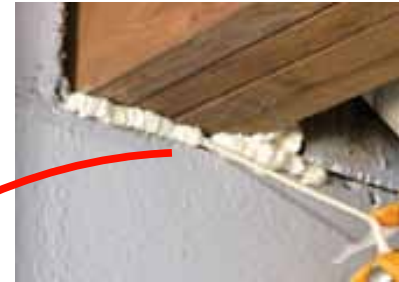
Ring of foam is applied to the gap between the drywall and the metal recessed fixture.
