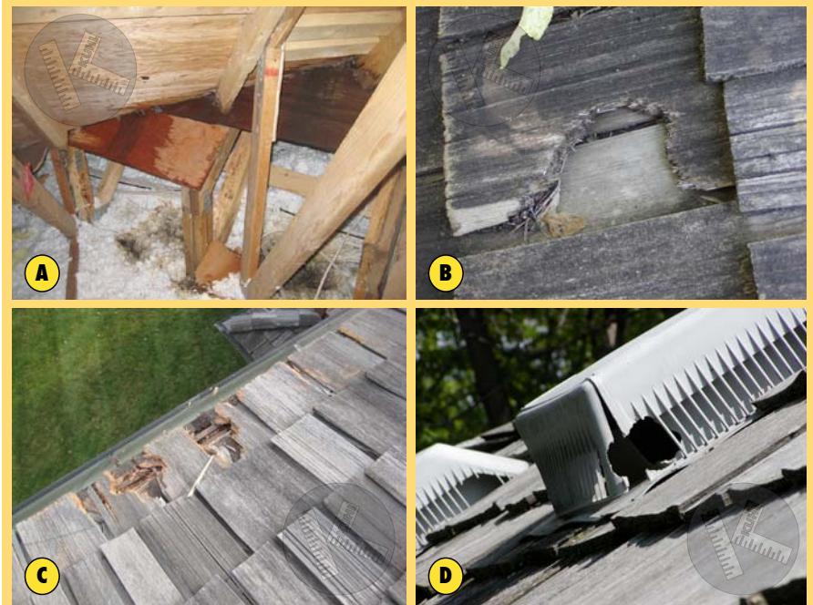
A - Massive leak in attic caused by squirrel. B - Cedar shake under assault by a squirrel. C - Two entry points for a family of squirrels. D - Roof vents with squirrel damage.
